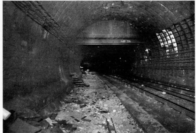
The site of North End's southbound platform with bridge taking subway to lower lift landing. Photo Nick Catford
